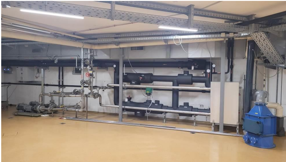
Figure 7: Brand new secondary cooling loop including new plate-type heat exchanger.
